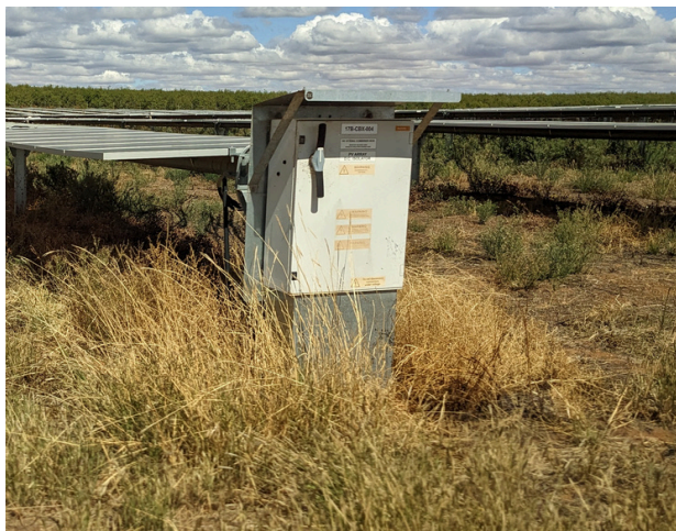
Unmanaged vegetation at string commander box.
